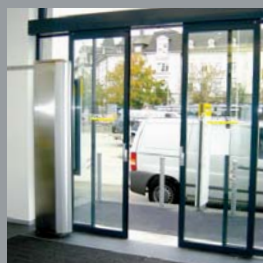
Installations for automatic sliding doors.
